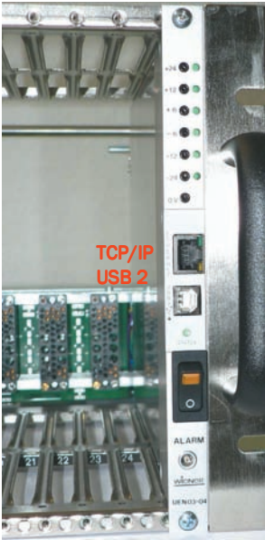
NIM control panel
